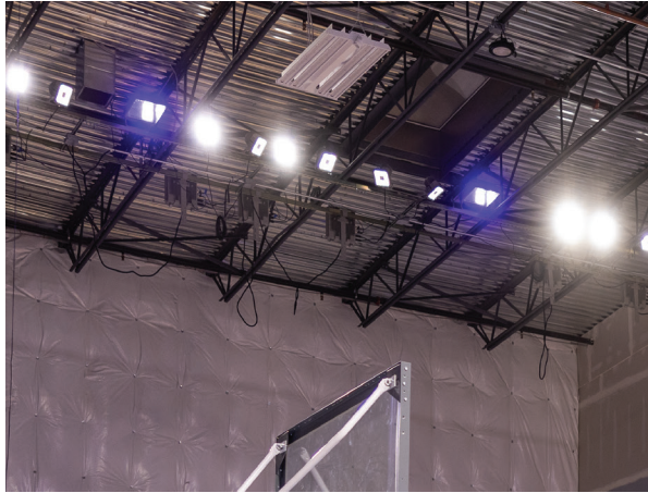
Sports field & gym lighting
